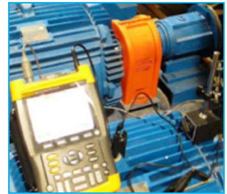
Before installation of AEGIS™ ring, two readings demonstrated the presence of damaging shaft voltages.
