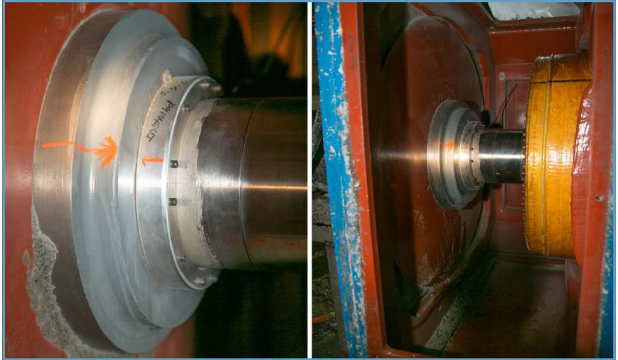
Close-ups of the AEGIS® PRO Bearing Protection Ring on a key motor in a Midwest paper mill. Prior to installation, the section of the motor shaft that would be contacted by the grounding ring's microfibers was thoroughly cleaned and coated with colloidal silver to enhance conductivity and retard corrosion.
