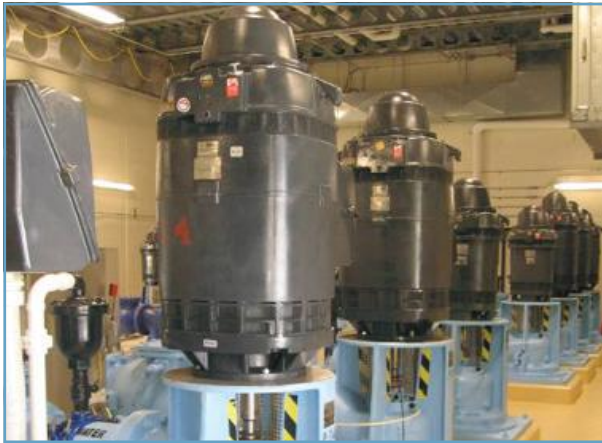
The motors atop these vertical hollow-shaft pumps (at the Reverse Osmosis Water Treatment Center in Hutchinson, Kansas) provide thrust to the pumps' drive ends.
