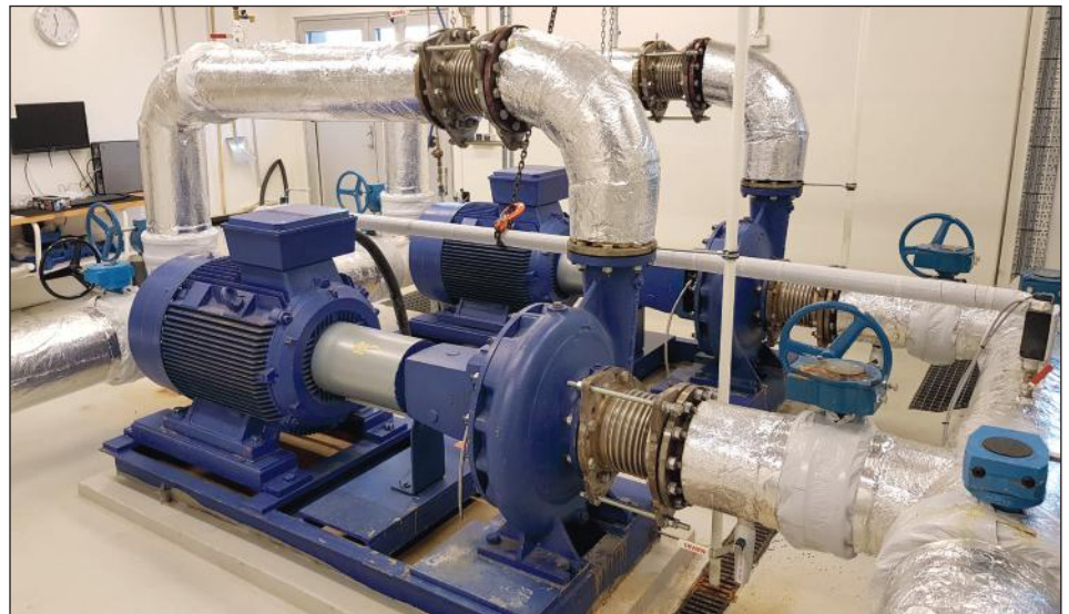
Geothermal heat pumps deliver water at a temperature of 70 degrees directly from the ground.
