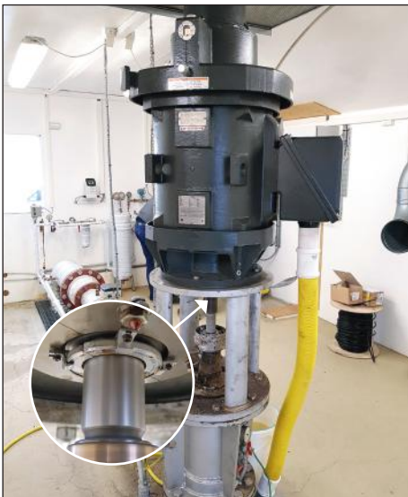
AEGIS® Split Shaft Grounding Ring installed on vertical deep well line shaft pump at a geothermal power station in Iceland.
