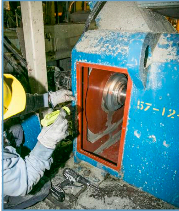
Inspecting the recently installed AEGIS® PRO Bearing Protection Ring on a key motor at the Midwest paper mill. Designed to close around the motor shaft, the split-ring PRO was installed without decoupling the motor.
