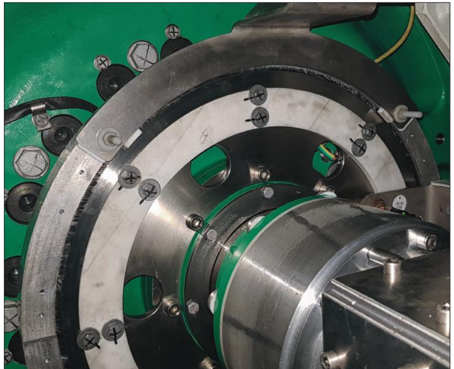
After installing the AEGIS® PRO ring, the shaft voltage could be reduced to less than one volt.
